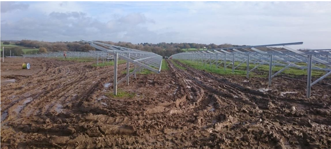
Photo 6: Panels Installed in Poorer Conditions
