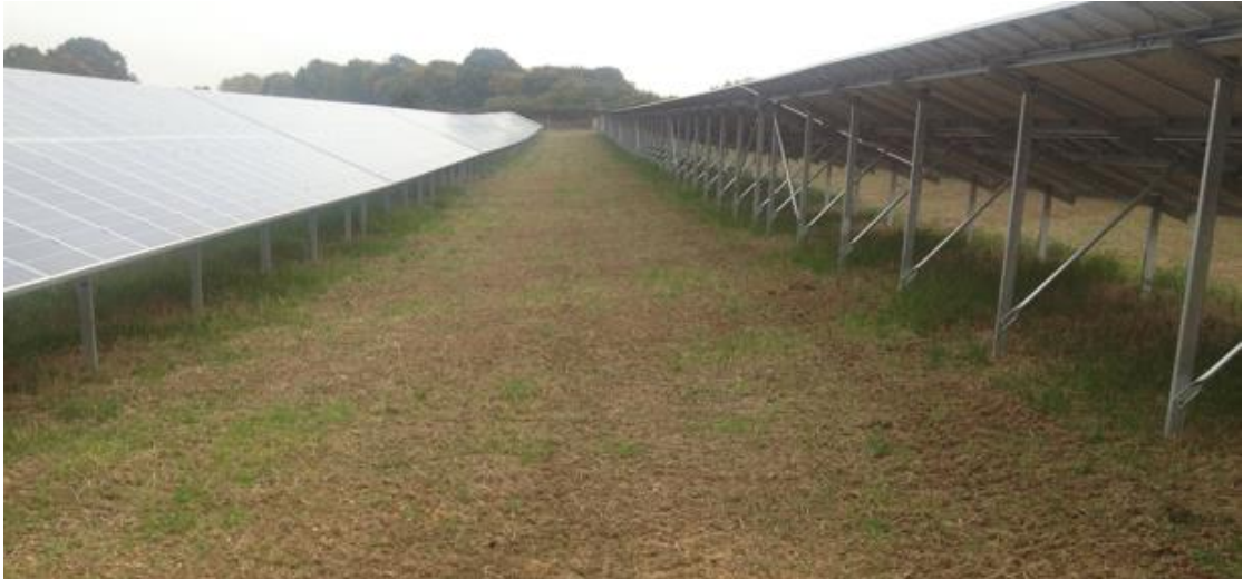
Photo 7: The Same Site Restored and Seeded (taken a few rows down from the previous picture)
