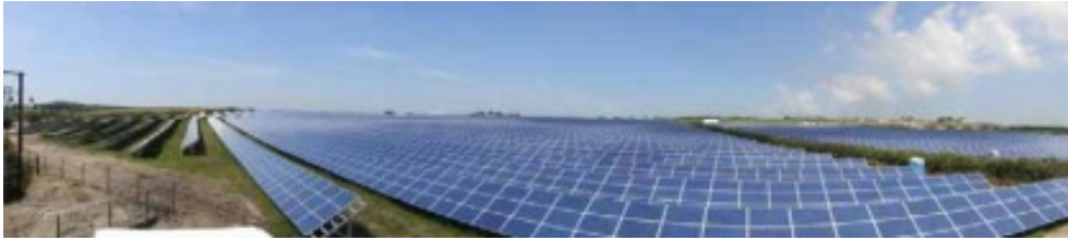
Solar PV facility adjacent to Saarbruecken airport.
