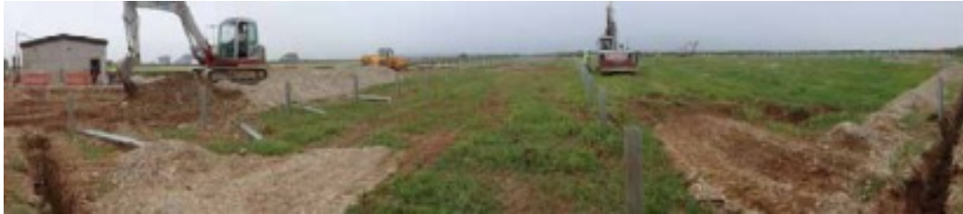
Development of the 5MW solar PV farm, Cornwall. Images courtesy of Low Carbon Solar Partners.
