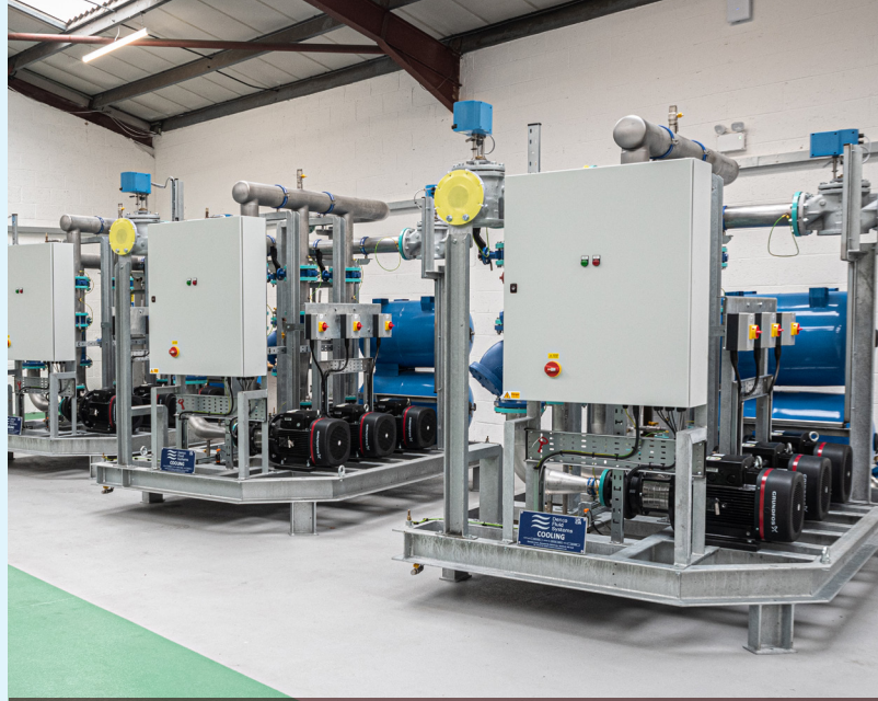
Denco's Pump Skid and Control Panel
