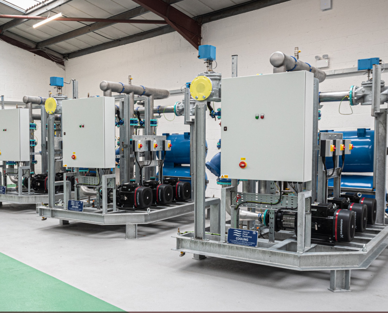
Denco's Pump Skid and Control Panel
